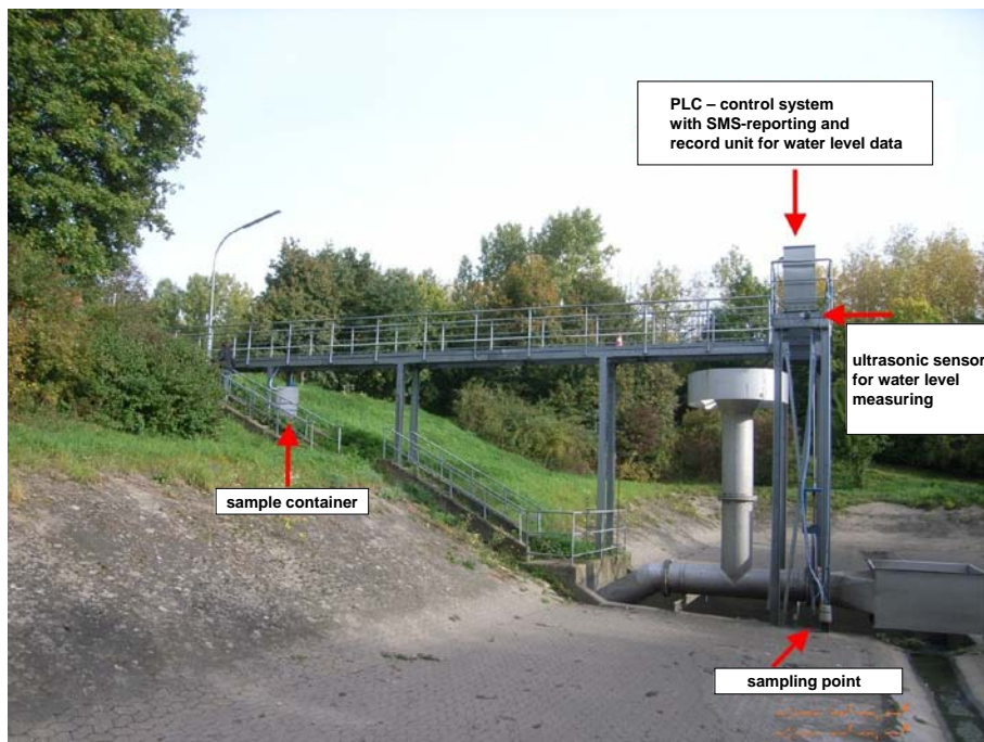
Figure 3: Stormwater retention tank – separate sewerage system Meckenheim site
